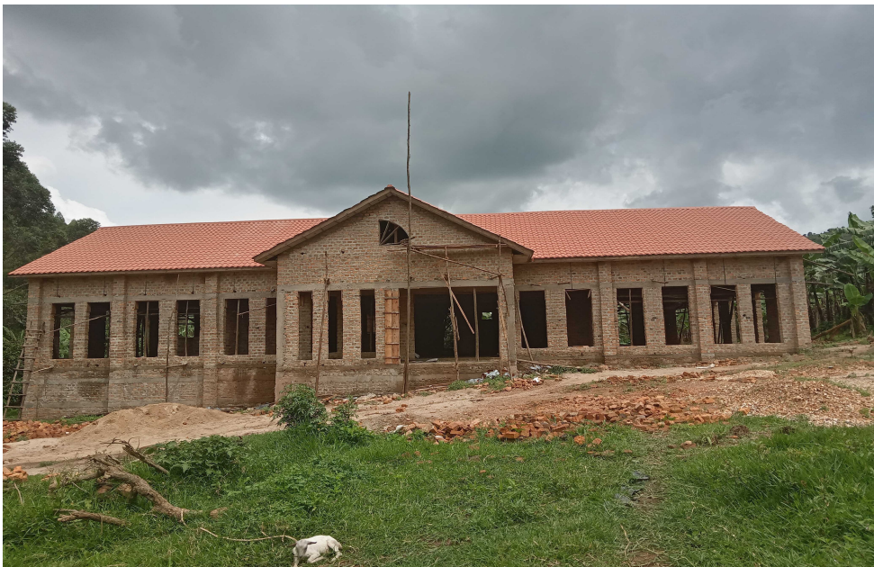
Fig 1: Current Status of the Library Structure
